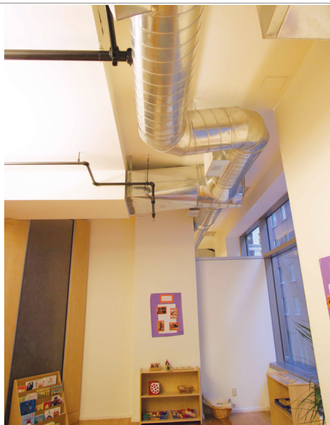
Ductwork, lighting, and a wet-type sprinkler system were part of Rand's design for the school's build-out.
